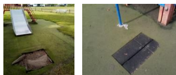
Austerity Bournemouth: Parts of Mallard Road Park playground's soft flooring are missing
