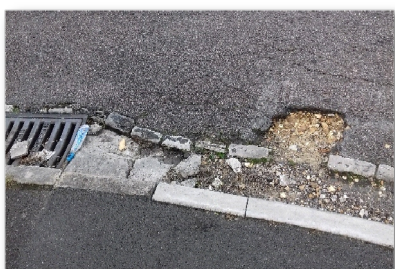
Potholes damage cars and make cycling dangerous
